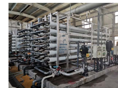
Figure: Extrusion washing wastewater treatment equipment of Jilin
